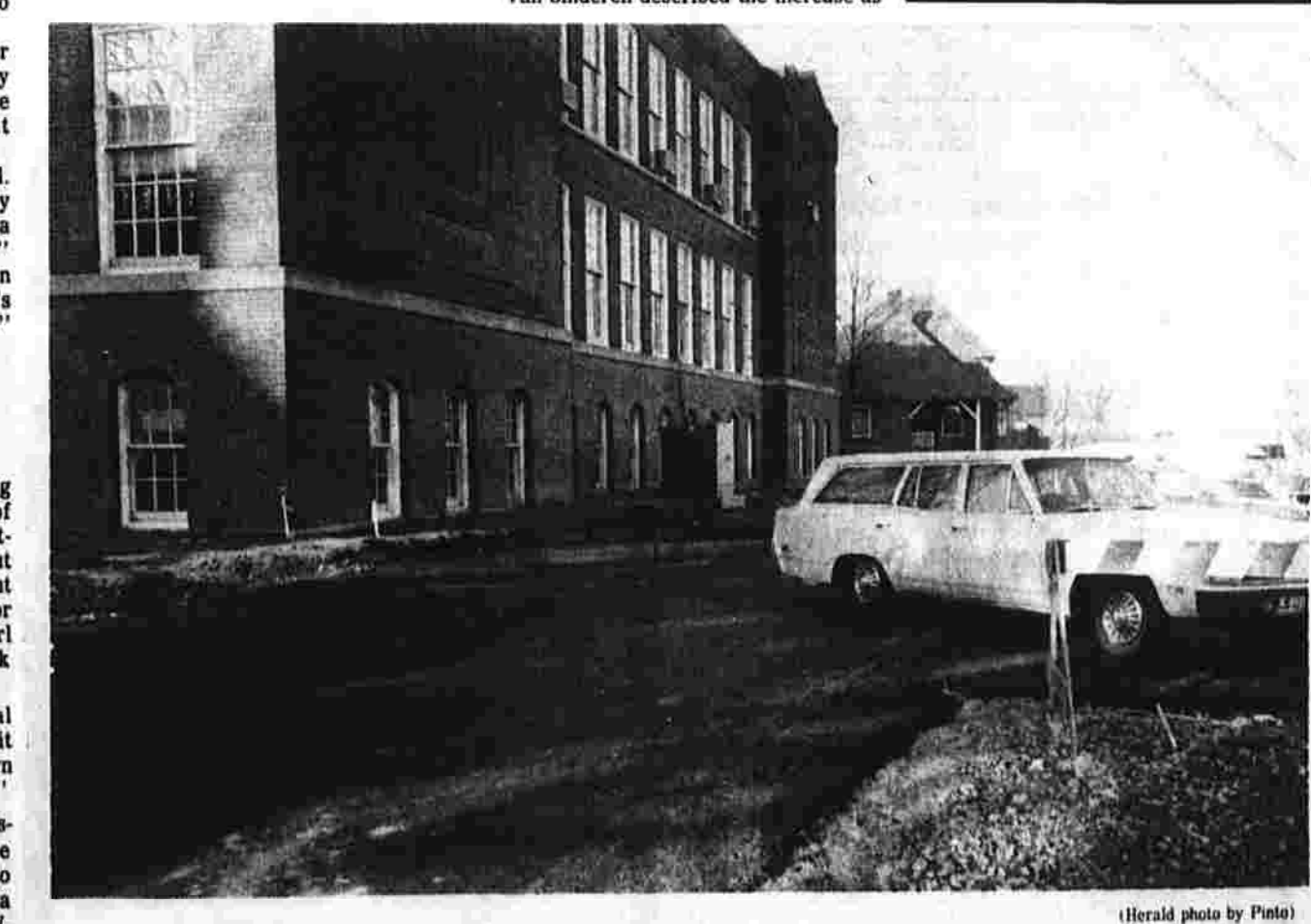
Controversial Driveway at Lincoln Center The Conservation Commission is voicing displeasure with the construction of this unneeded driveway and parking area along the Main St. side of Manchester's Lincoln Center. It is part of the plan for improving access and entry for employees and visitors. When the project is completed, cars will enter from Main St. only at the north end of the building. The existing driveway, at the traffic light at E. Center St., will be filled in, landscaped and closed. The new driveway will turn right at the south end of the building, then will turn right again, winding around Lincoln Center to the Municipal Building parking lot.
